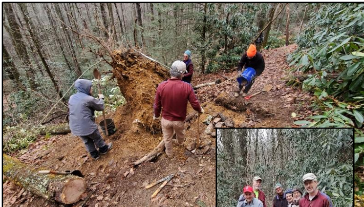
Typical MRATC workday – repairing tread after uprooted tree damaged the trail – Dickey Gap. From left to right, Randy Goodman, Ron Bobko, Sharon Trumbley, Anne Maio, Jim Wilson, and Doug Levin.
